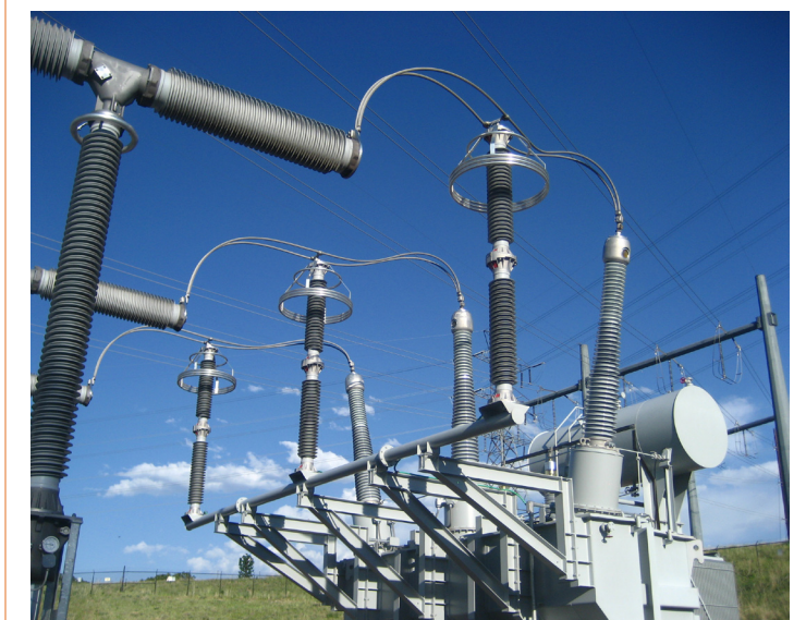
Above: Addition of properly located surge arresters gives protection to the E1 and E2 portion of the EMP spectrum
